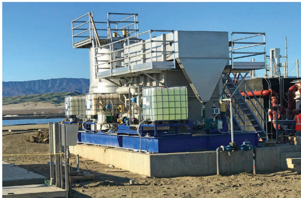
The skid-mounted Suspended Air Flotation unit (Heron Innovators) creates fine bubbles using a froth generator.
