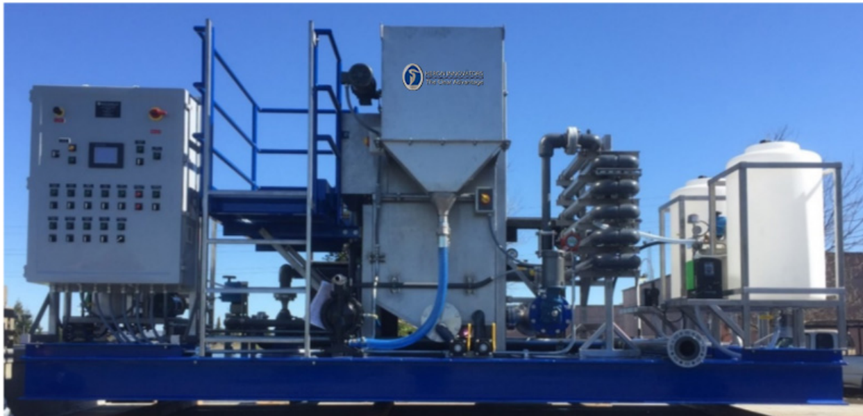
Figure 4. Suspended Air® Flotation Process – Entire Skid Mounted Water Treatment System; Inclusive of SAF Generator, Clear Floater, Serpentine Style Mixing Chamber, Chemical Staging, Polymer Mixer/Aging System, Floccmixer, Flowmeters, Solids Hopper, Pumps, PLC Cabinet and Maintenance Platform. (8' x 16' skid can accommodate up to 1,000 gpm)
